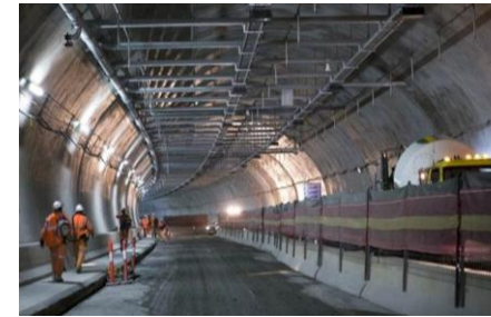
Eastlink Tunnel Melbourne, Australia
